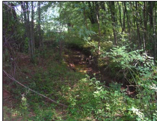
Eroded Outlet at Union Township Middle School
